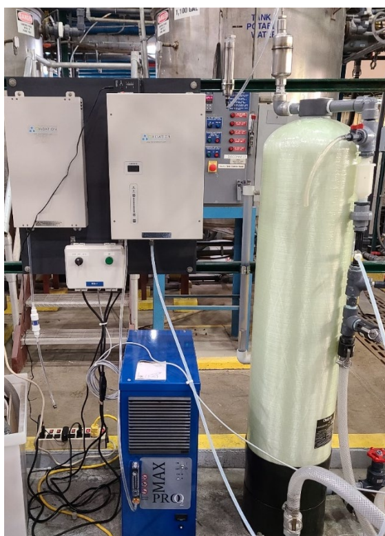
Figure 4. O 3 system (air dryer, oxygen generator, O 3 generator, contact tank)
