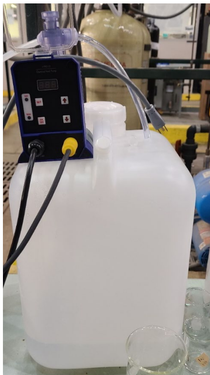
Figure 3. H 2 O 2 injection system
